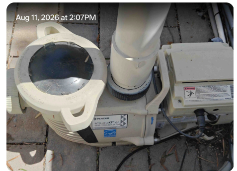
Pump P-2: Pentair IntelliFloXF VSF variable-speed and flow pump.
