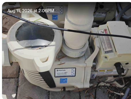
Pump P-1: Pentair IntelliFloXF variable-speed pump.
