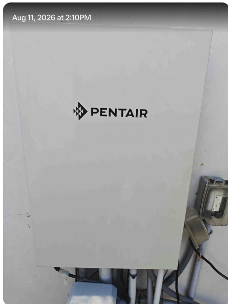
Existing older-generation automation equipment.
