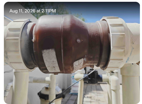
Leak 3 at the large 4-inch swing check valve.
