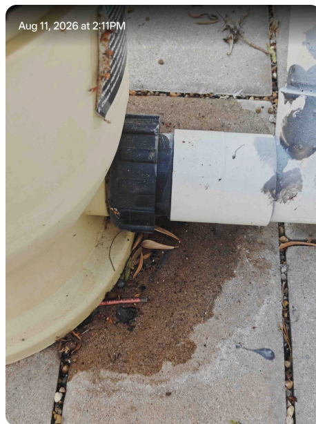
Leak 2 at the smaller Clean & Clear filter union.
