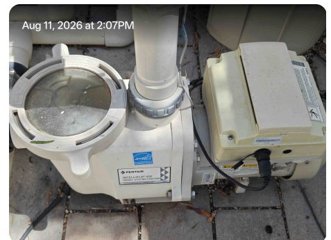
Pump P-3: Pentair IntelliFlo VSF variable-speed and flow pump.
