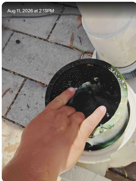
Visible algae and organic accumulation in an affected pump basket.
