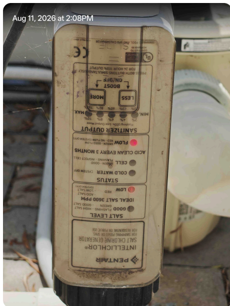
Sanitizer S-3: Pentair IntelliChlor salt chlorine generator.
