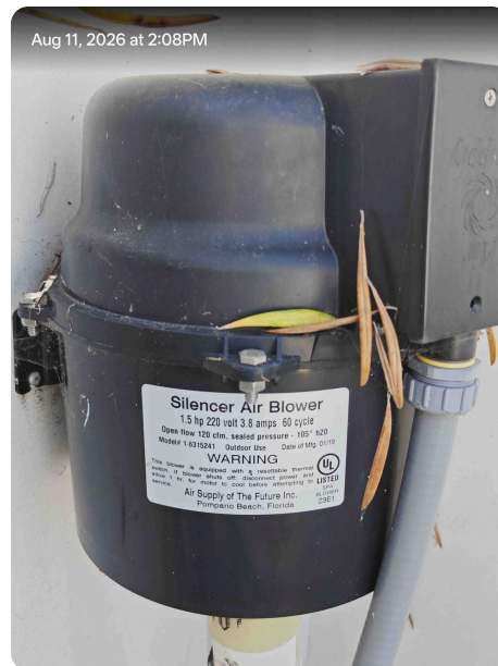
Air blower B-1: Silencer 1.5 HP blower, manufactured January 2019.
