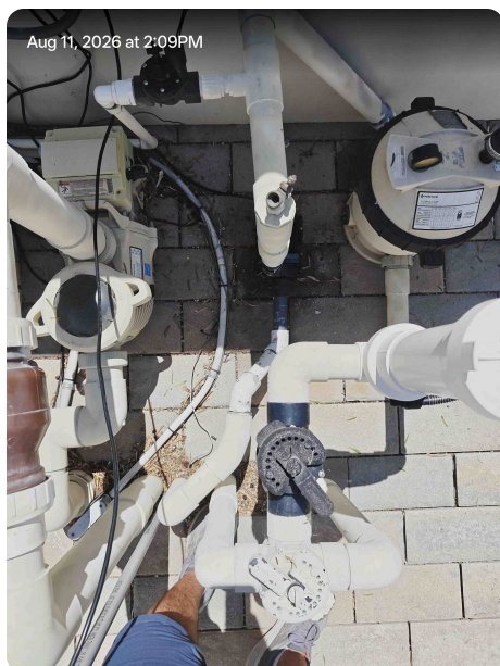
Leak 1 at a union connection.
